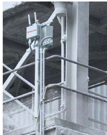
Wiring is a chronic weak point close to a harsh steel furnace.
