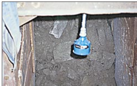
Monitoring levels in a limestone crushing process.
