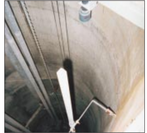
Reliable dual-pump control in a narrow lift station with obstructions.
